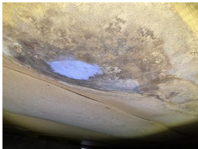
Fuktfläck under pannrum/badrum i krypgrund.
