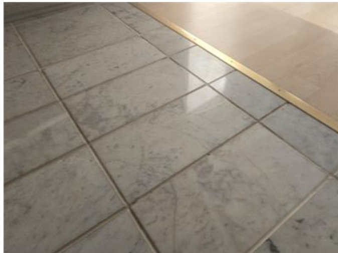
Spruckna klinkerplattor, entréhall.
