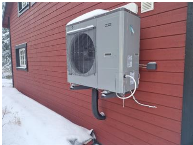
Luftvärmepumpens ute del.
